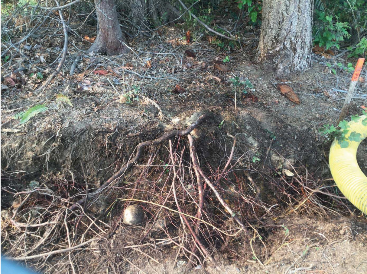
Photo 2. Exposed roots from the Hydrovac adjacent to #7337. Dense mat of feeder roots with medium sized lateral roots. The cut to occur within less than a meter from tree 7337 would de-stabilize the tree.
