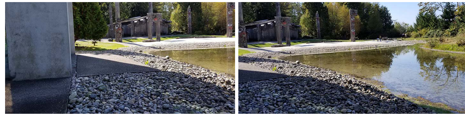
Views G23 Sheet L4 (G23:L4) existing site conditions | grading | cobbles | pea gravel at pond edge | aggregate concrete pads | vegetation
