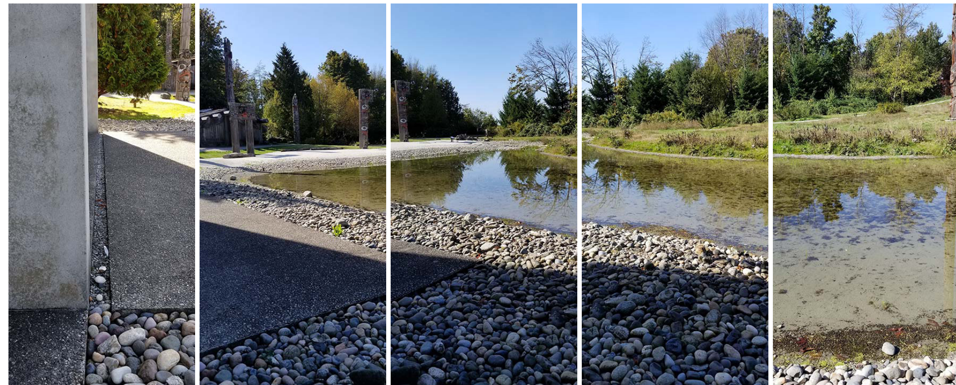
Views G23 Sheet L4 (G23:L4) existing site conditions | aggregate concrete | cobbles | grading | pea gravel at pond water's edge | vegetation
