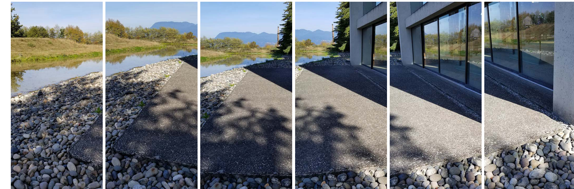
Views G19 Sheet L4 (G19:L4) existing site conditions at large aggregate concrete pad west side of Great Hall | grading | cobbles | concrete interface with glazing
