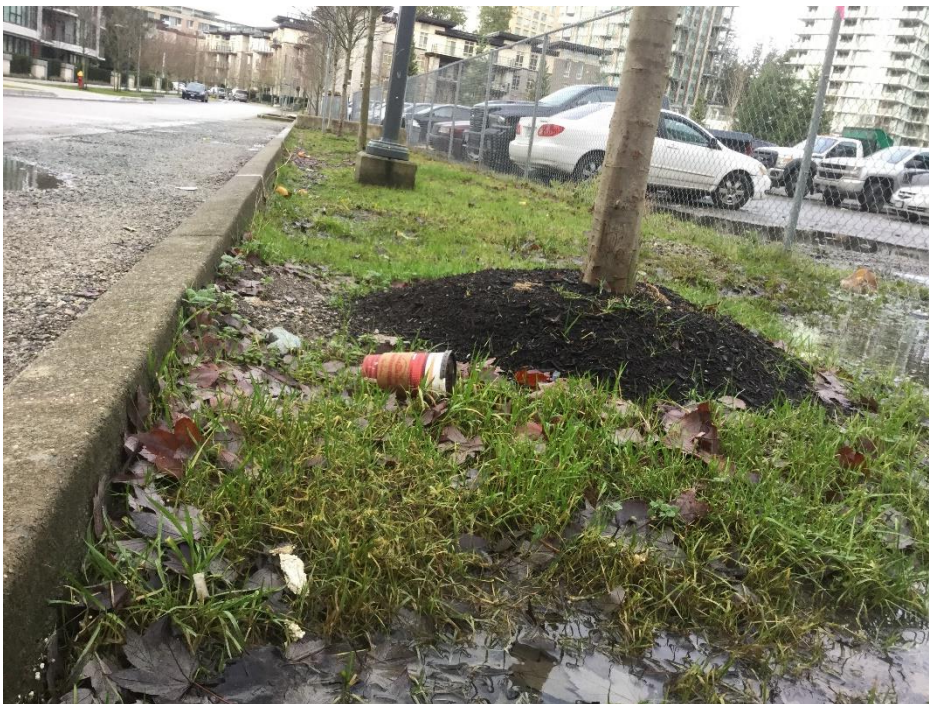
Photo 4. Street trees on Birney Ave have been planted proud. There is good opportunity to improve growing conditions in the boulevard.
