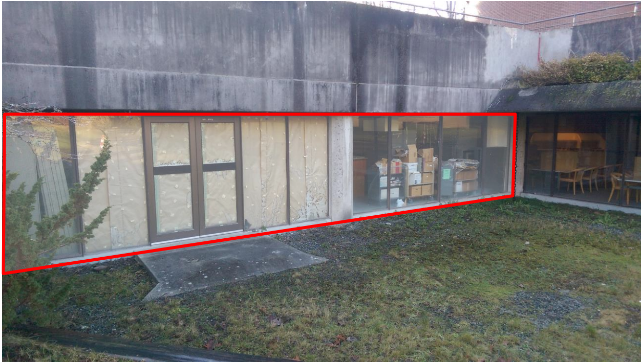
Photo 5: Below portion of the Site. The area consists of several rooms of the Walter C. Koerner Library.
