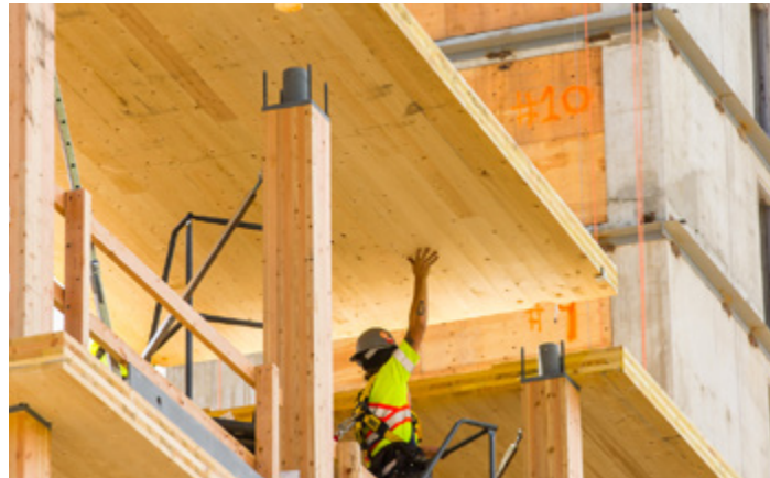
Mass timber construction at Brock Commons Tallwood House. (Photo Credit: KK Law)
