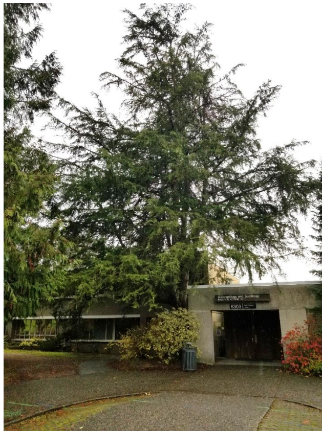
Photo 4. Tree #1707, Tree planted right against existing building. Viewing northwest.
