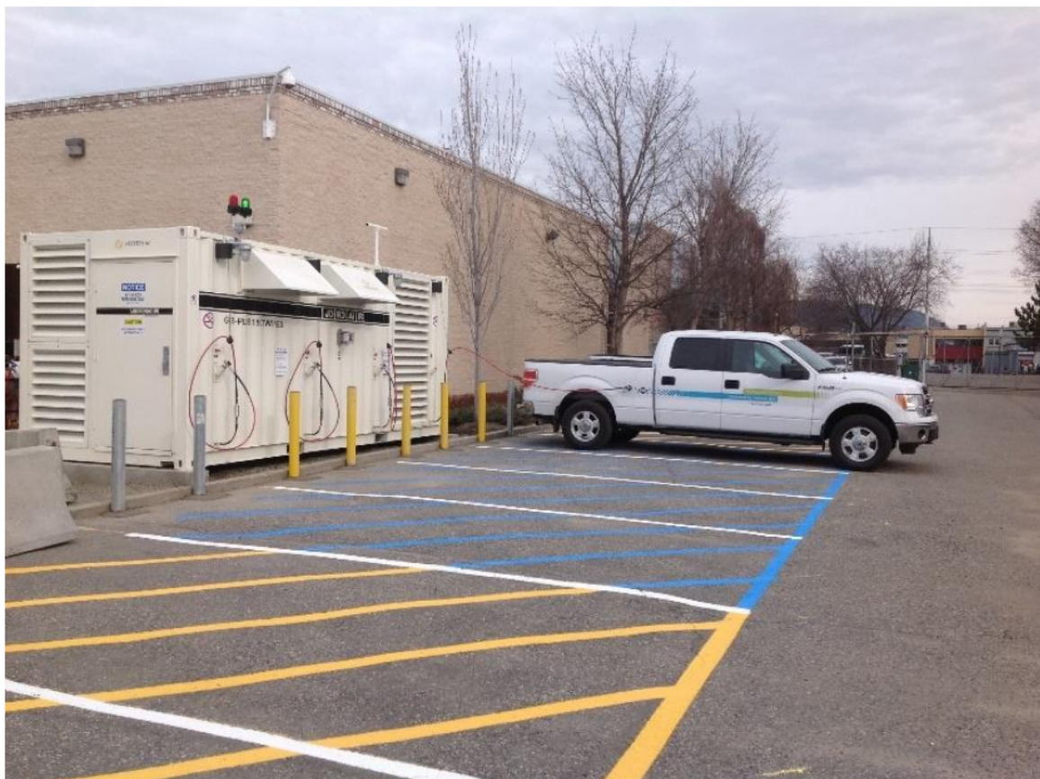
15 JORDAIR NGV DUPLEX GAS-PACK FUELING SYSTEM
